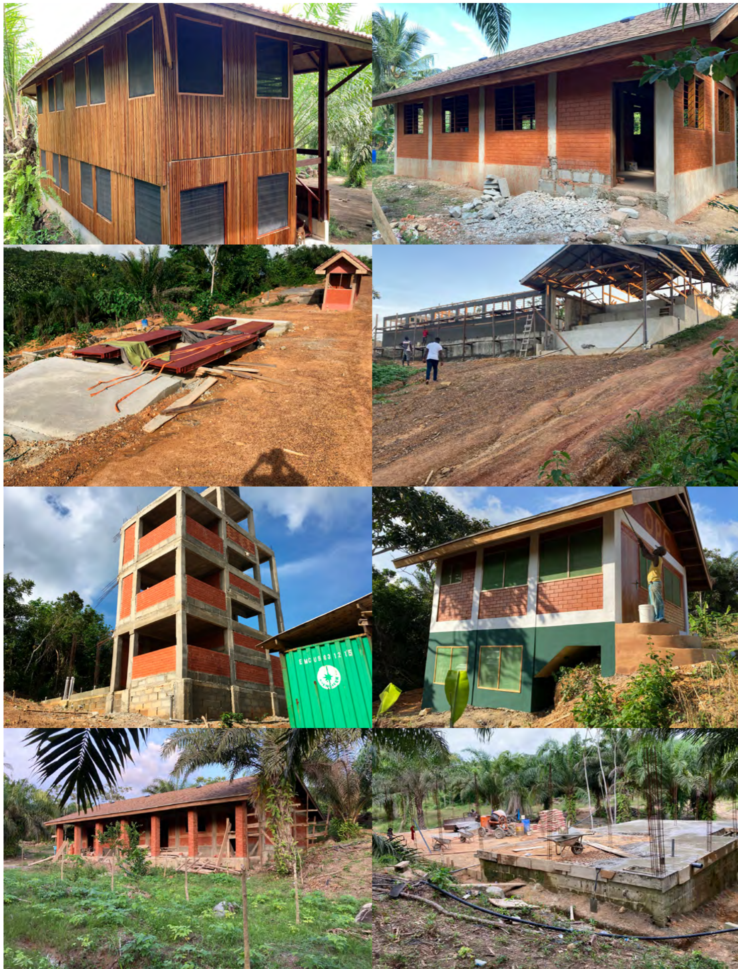
Impressions of the construction in Busua; residential house and herbal clinic (top), weighbridge and gate house, as well as mill for sustainable palm oil and soap factory (upper middle), staircase guesthouse with main distribution tank and administration building (lower middle), school and foundation event centre (bottom).
