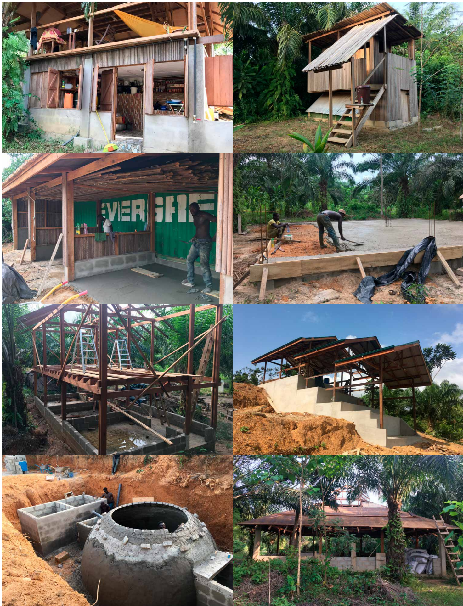
Impressions of the construction in Busua; kitchen and compost toilet (top), workshop and foundation of the food processing centre (upper middle), foundation & woodwork of the residential house, mill for sustainable palm oil (lower middle), biogas plant and roof work food processing centre (bottom).
