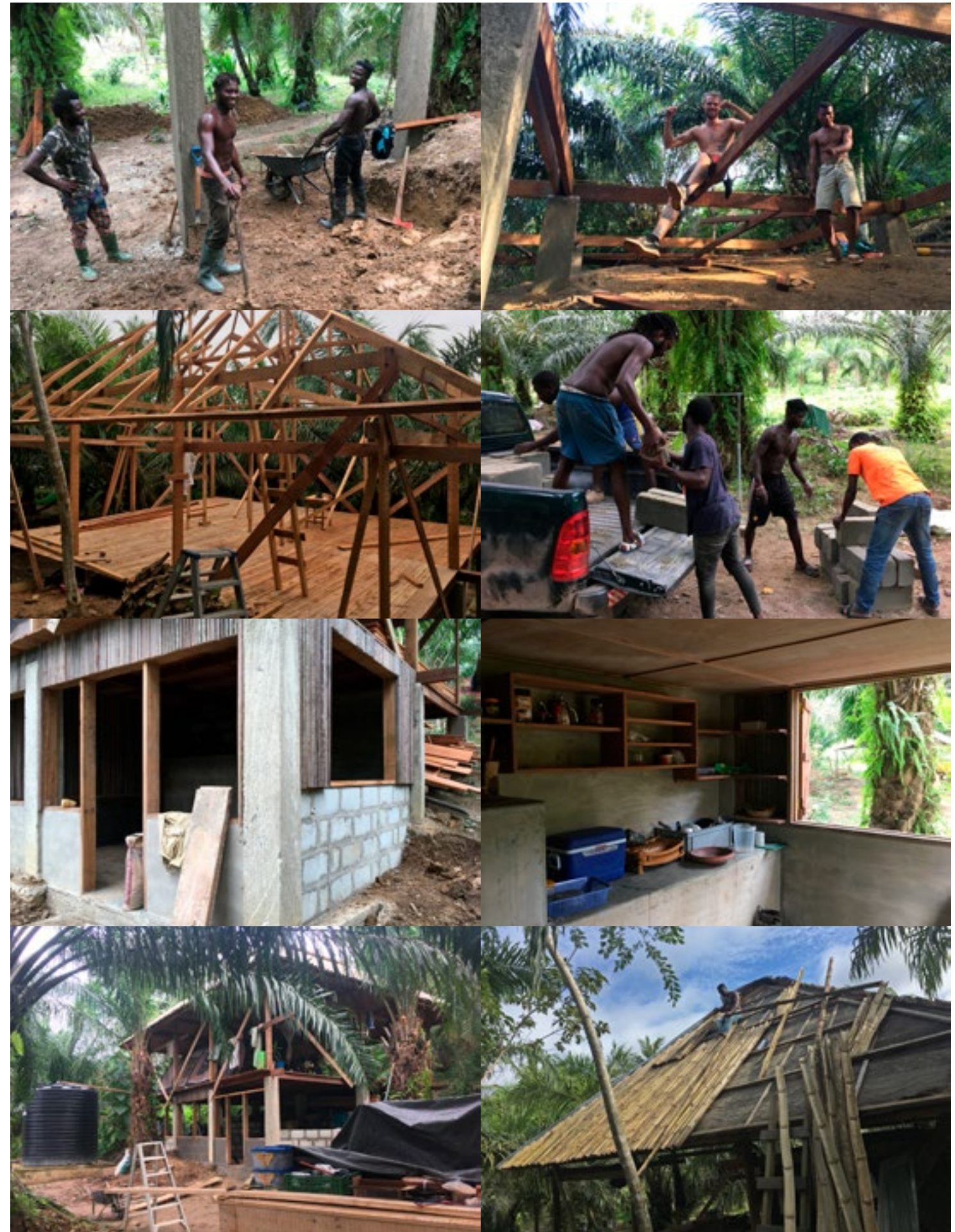
Impressions of the construction of the wooden platform, which has meanwhile developed into a three-storey building with kitchen, storeroom, platform and mass sleeping area
